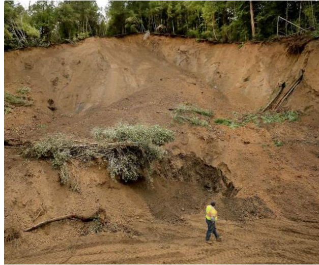
Engineered slope failure in Sonoma Co. after late Feb 2019 storm PC: Press-Democrat
