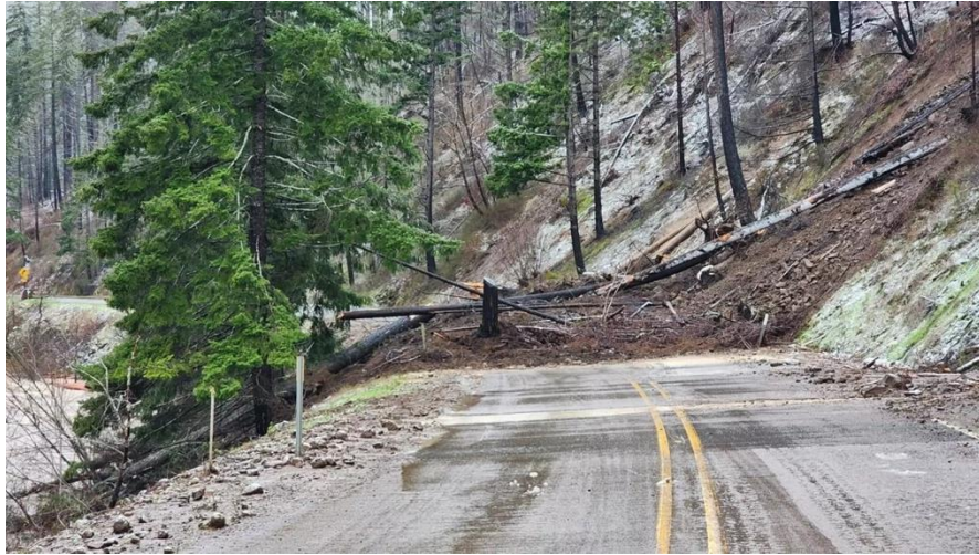
Slide on Highway 138 in Douglas County
